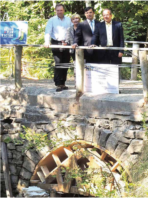
HERITAGE BRIDGE – Ted Arnott, Councillor Joan Robson, MP Michael Chong, and Halton Hills Mayor Rick Bonnette look at the progress being made on the restoration of the heritage bridge on 27th Sideroad north of Georgetown. The bridge dates back to the 1870s.
